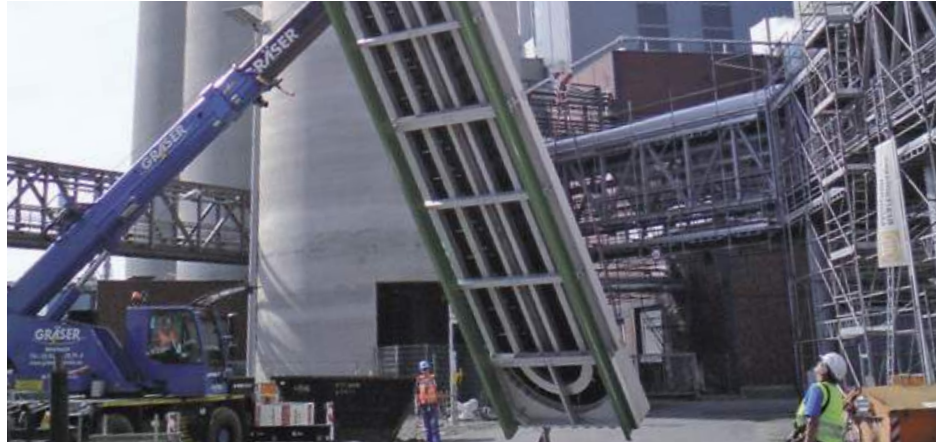
MultiDisc® Installation at the GKM Power Plant in Mannheim
